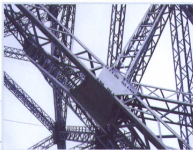
Power Transmission Line 220KV
