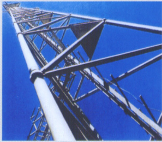
Power Transmission Line By Steel Tube Tower
